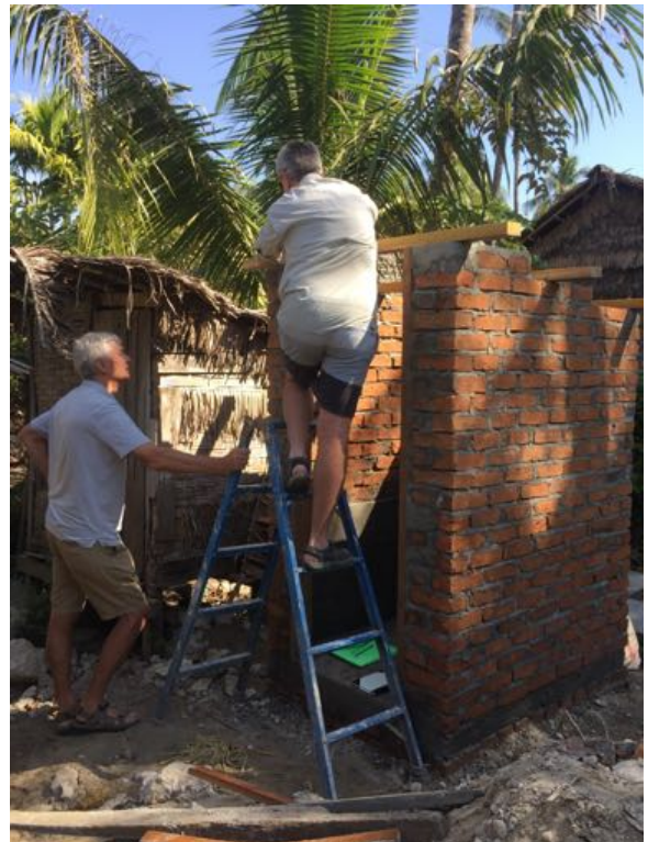
Robin and Brant check requirements for the roof and door to complete the toilet.
