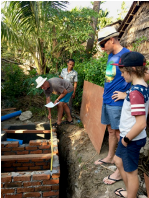
Htein Lin with Jamie measuring the septic tank with Tim and Luke supervising.
