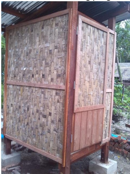
The new toilet with iron roof, bamboo walls and squat pan and septic tank.
