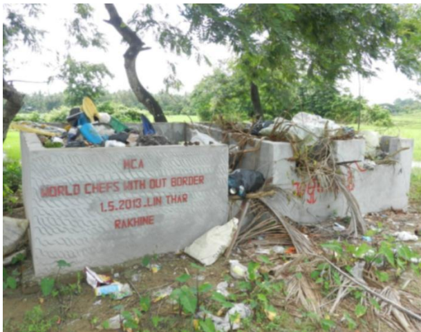
Efforts by Chefs Without Borders to build concrete bunkers for waste and recycling but no method or system to empty the bunkers
