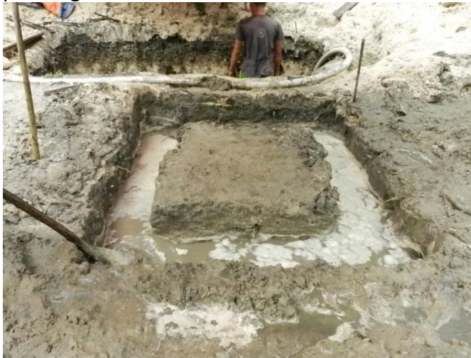
Miscommunication resulted in toilet foundations being over excavated.
