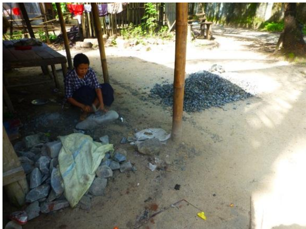
Local villager crushing stone with a hammer to make blue metal for outlet pipe bedding.
