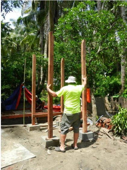
Corner posts for the toilet in position. The sun is out – but not for long!!
