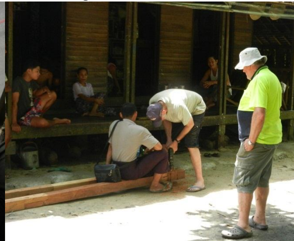
Using the only power drill at a nearby home with locals watching.
